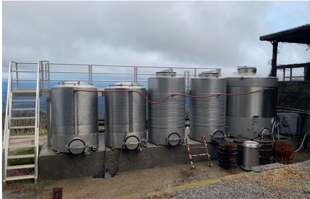
These steel tanks were used for the Pinot Noir until 2008
